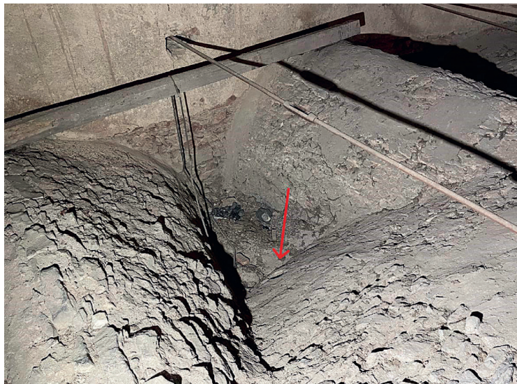
Fig. 10. Church of Saint Adalbert in Jílové u Prahy, vault of choir with a vessel marked by an arrow (photo by F. Facincani).
